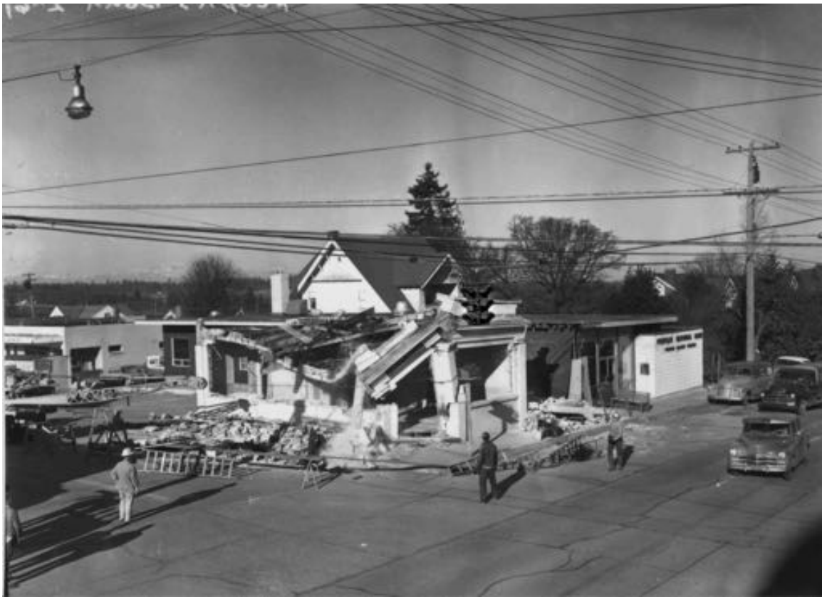
Demolition of Vashon State Bank New People's National Bank Building behind, 1961 Courtesy of the Vashon-Maury Island Heritage Museum
